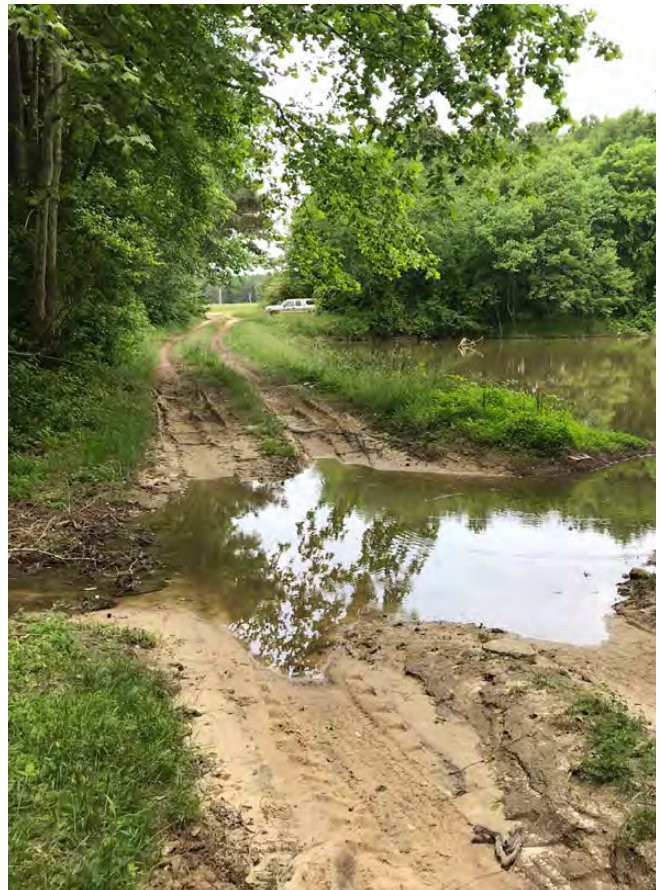
Figure 18: Current condition of a dam on the park property
