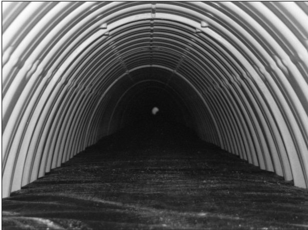
Looking down the Isolator Row from the manhole opening, woven geotextile is shown between the chamber and stone base.
